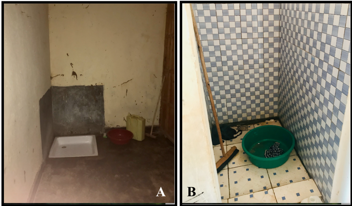
Figure 7. WASH facilities in MHM rooms. A. WASH facilities in a public school. Jerry can and bucket contained water for washing, mop present to clean facilities. Smears of menstrual blood and fecal matter can be seen on the wall. B. WASH facilities in a government aided school. Water and soap were present in a bucket outside the shower stall. Mop and wash basin present for cleaning the facilities. Photos: Kirsten Dodroe, with permission.
